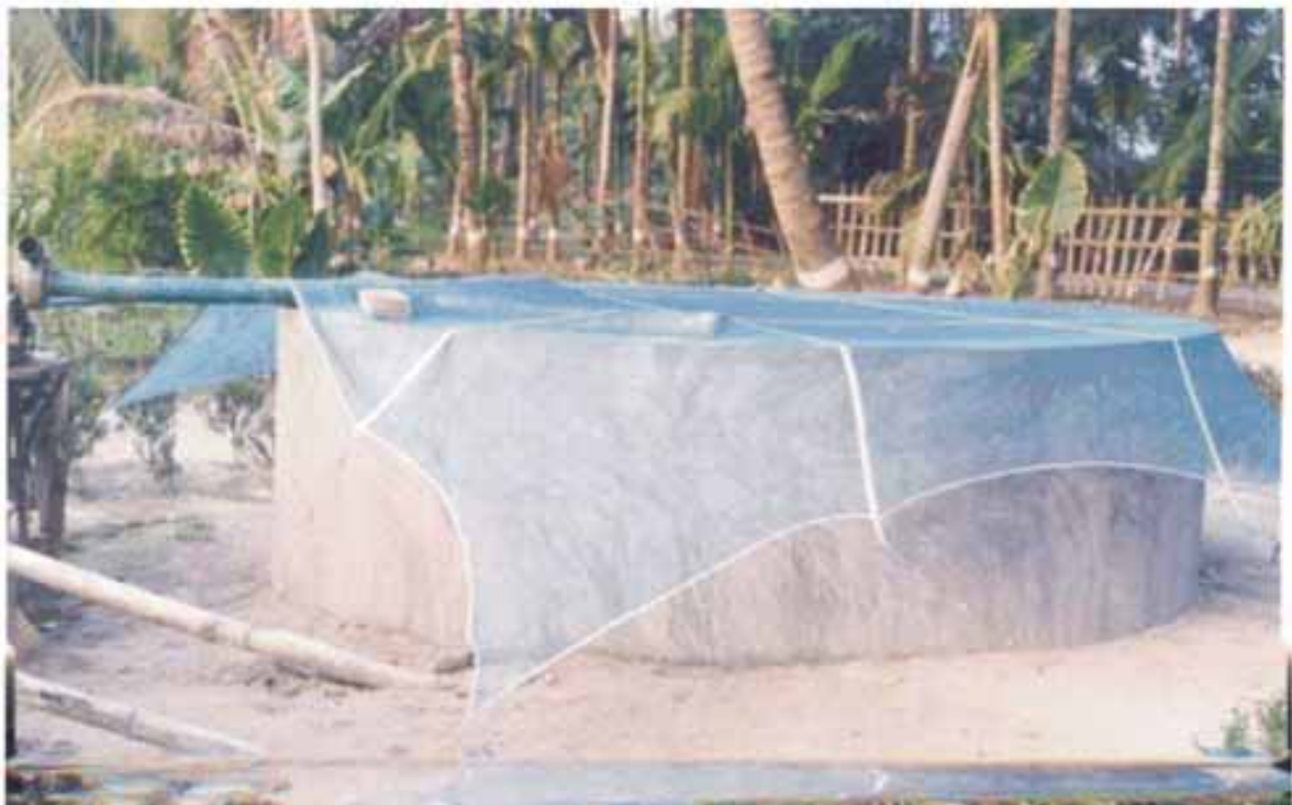
Figure 10(d): The complete dugwell just after construction covered with mosquito net (to prevent surface contamination).
